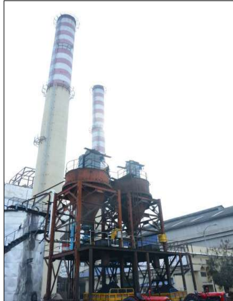
Boiler Ash Handling System
